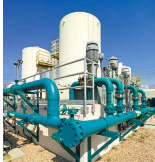
The Edward C. Little Water Recycling Facility has produced more than 200 billion gallons of recycled water.
