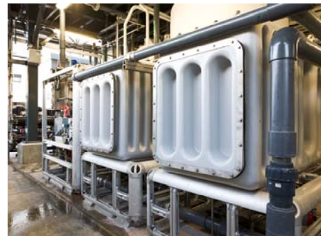
This Ultrafiltration unit at the NEW Desalination Demonstration Facility in Redondo Beach is the first step in desalinating ocean-water.
