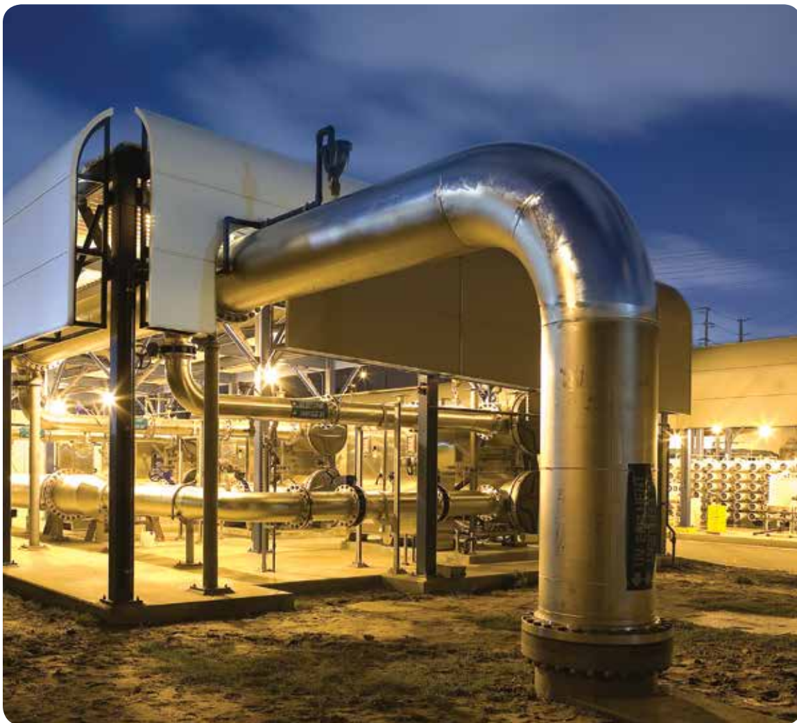
Edward C. Little Water Recycling Facility
