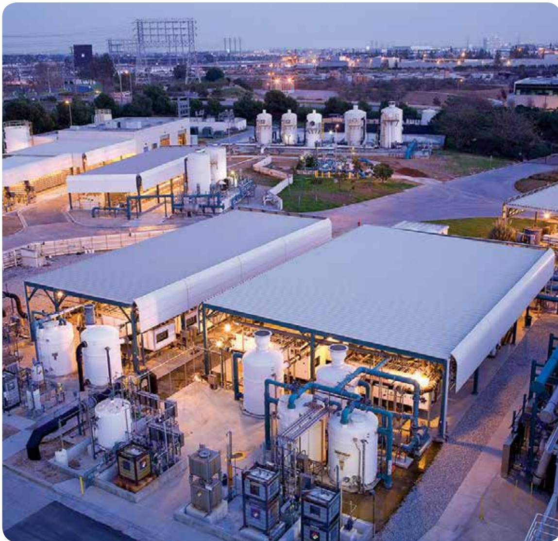
Edward C. Little Water Recycling Facility
