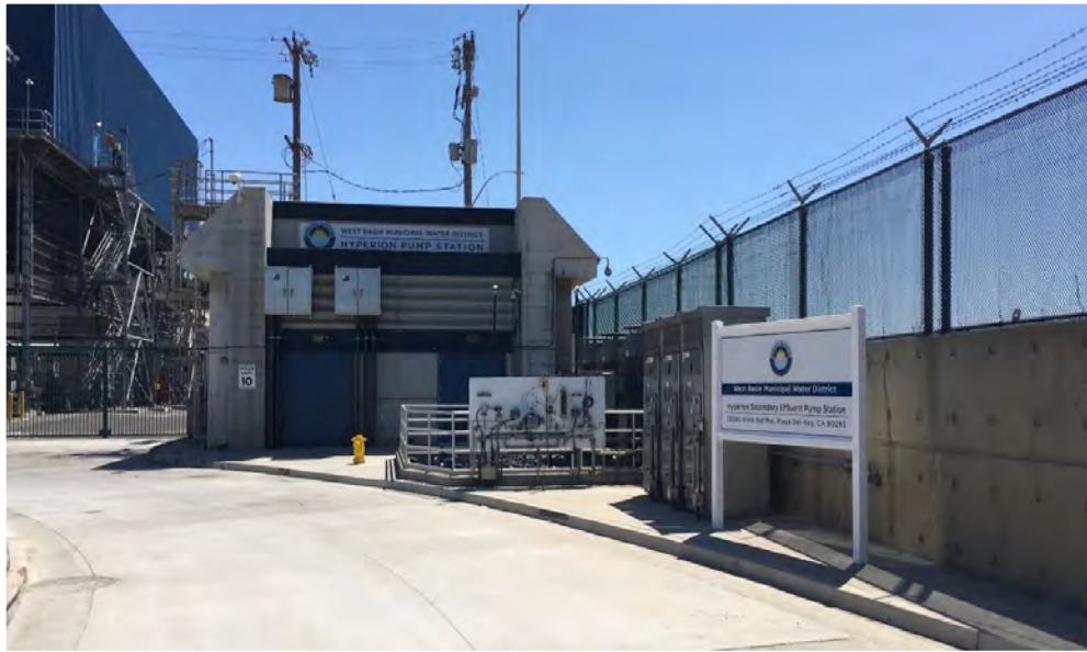
Existing Hyperion Pump Station (Indoor) alongside New Pump Station (Outdoor)
