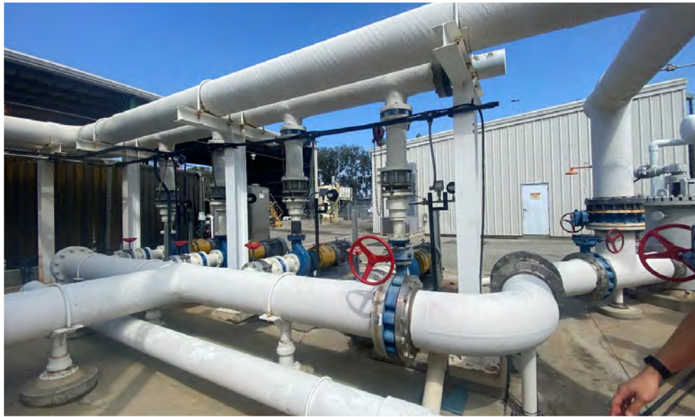
TRWRP Fiberglass Pipeline upstream of the cartridge filters
