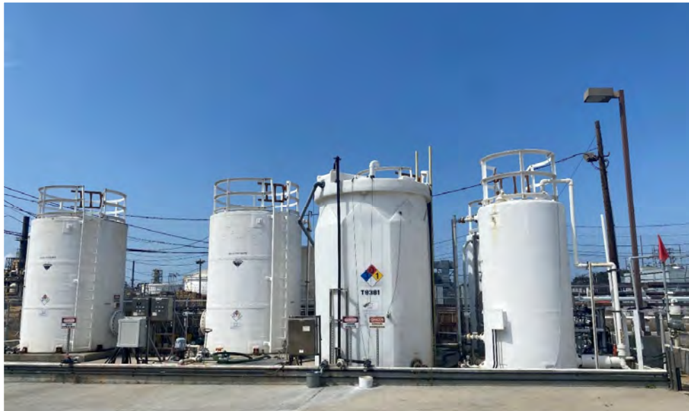
Bulk Chemical Storage Tanks at TRWRP
