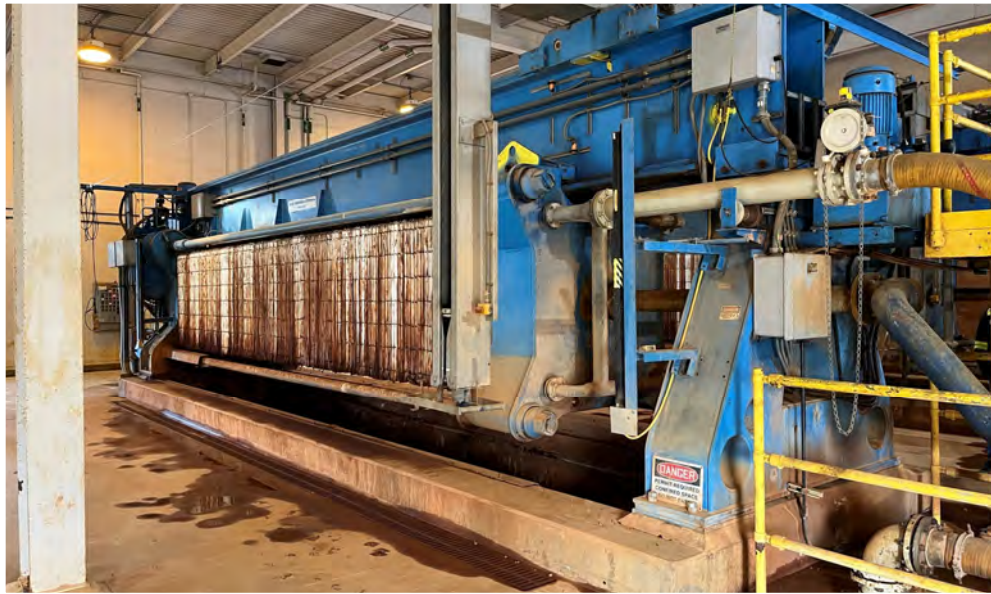
Plate and Frame Filter Press #1 in the Dewatering Building at ECLWRF
