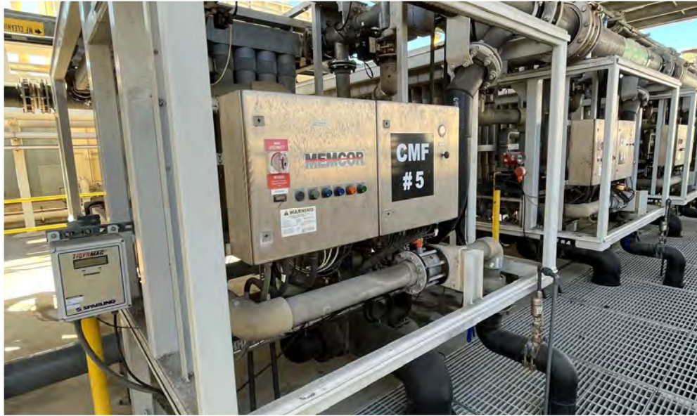
A local programmable logic controller (PLC) at Torrance Refinery Water Recycling Plant
