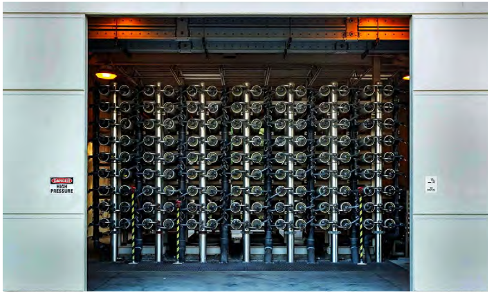
Reverse Osmosis Membranes at ECLWRF
