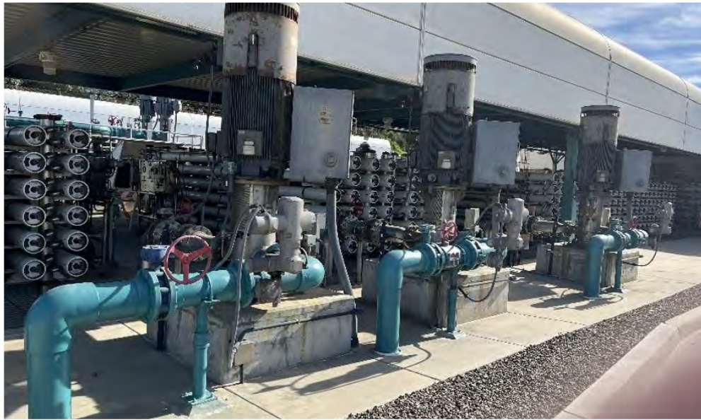
RO Feed Pumps
