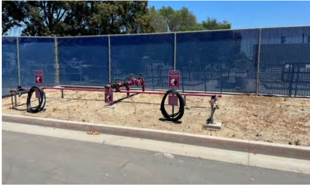
Los Angeles Department of Water and Power Commercial Fill Station
