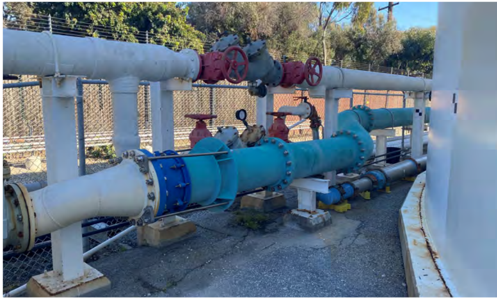
Existing Backflow Preventer
