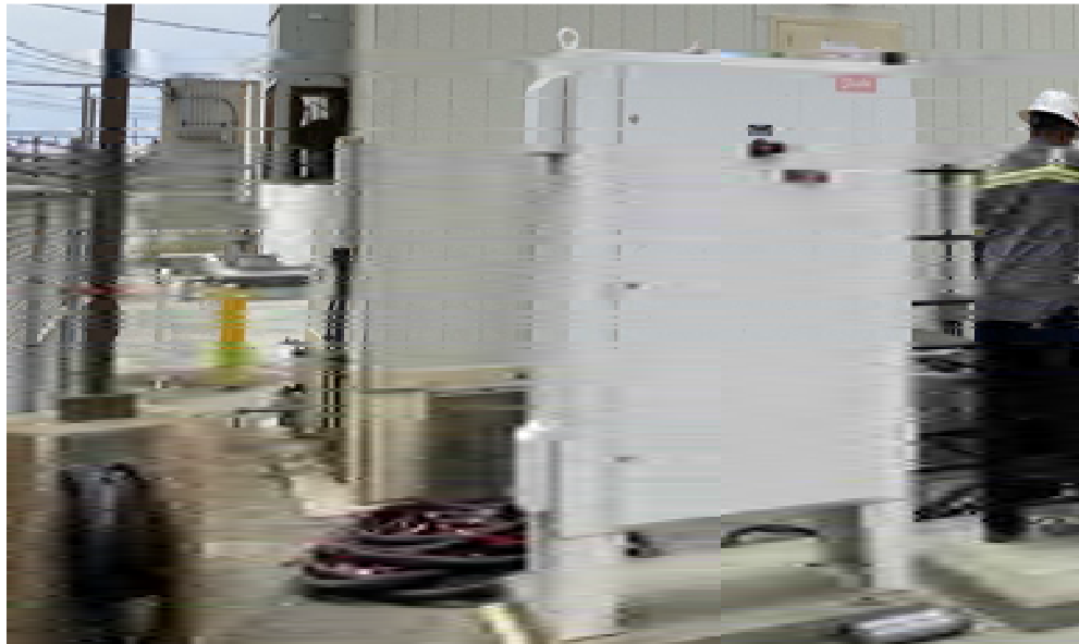
Motor control center at TRWRP.
