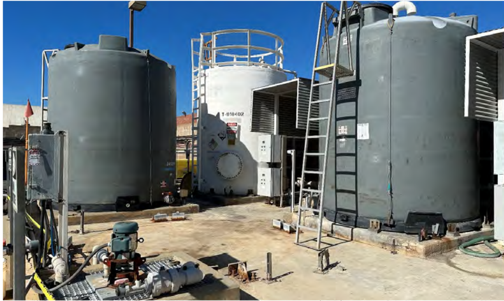
(2) Temporary 6,900-gal Rain For Rent sodium hypochlorite tanks (grey) and existing 7,985-gal sodium hypochlorite tank (white) at CNTP
