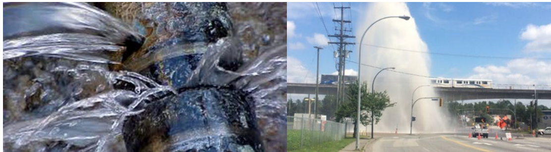
Figure 7-10. Pipe Breaks with Low Pressure (Left) and High Pressure (Right)
